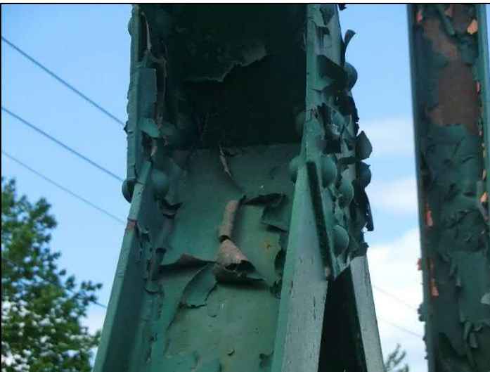
Figure 5. Peeling paint and Crevices in Route 102 Bridge
