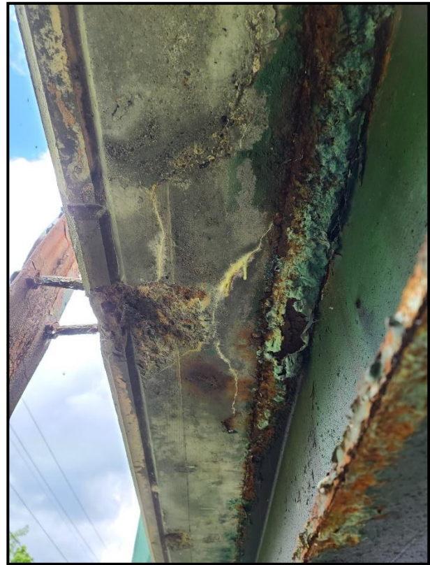
Figure 1-11: Deck Deterioration in Overhang
