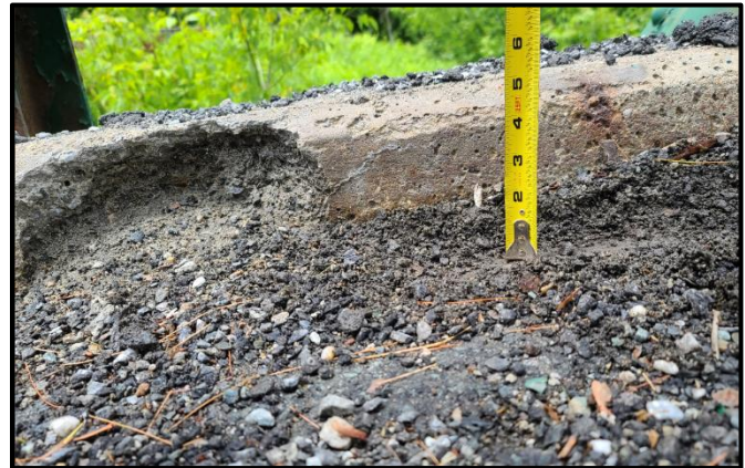
Figure 1-10: Spall in Curb
