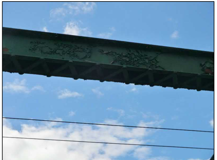
Figure 6. Peeling paint and crevices in Route 102 Bridge
