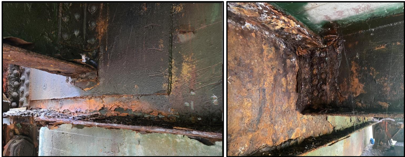
Figure 1-7: Expansion End Floor Beam Condition
