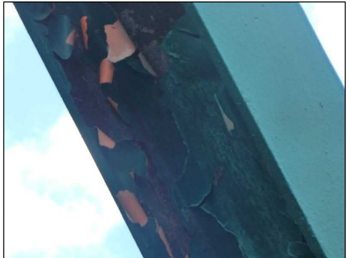
Figure 4. Peeling paint in Route 102 Bridge
