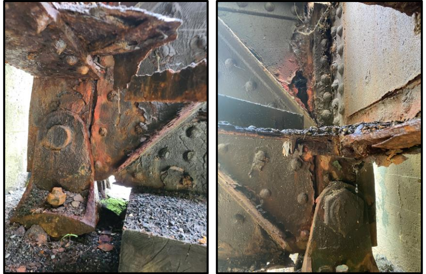
Figure 1-8: Severe Deterioration of End Bearings, Plates, and Connections
