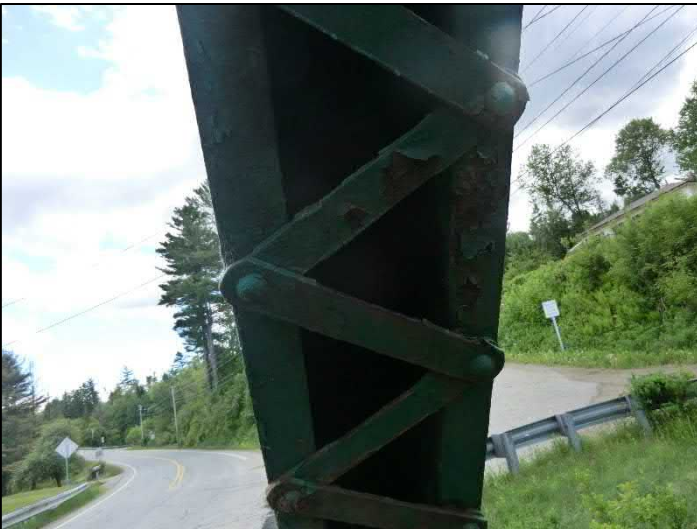
Figure 3. Crevices in Route 102 Bridge
