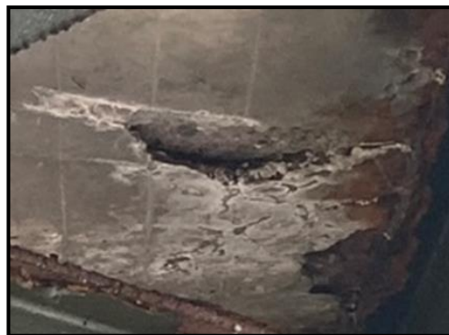
Figure 1-13: Spall in Underside of Deck
